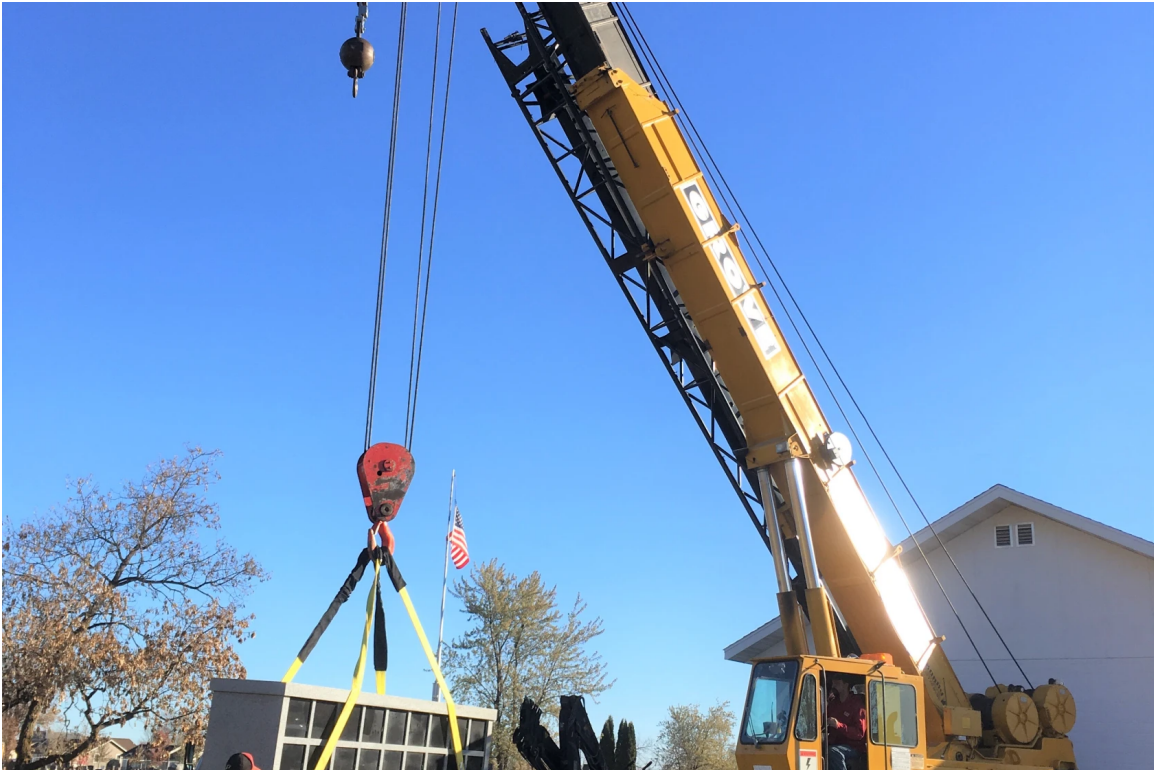
1/2: A crane sets the columbarium in place on a concrete pad while three men line it up Monday, Oct. 22 in the Wadena Cemetery. Michael Johnson/Pioneer Journal
