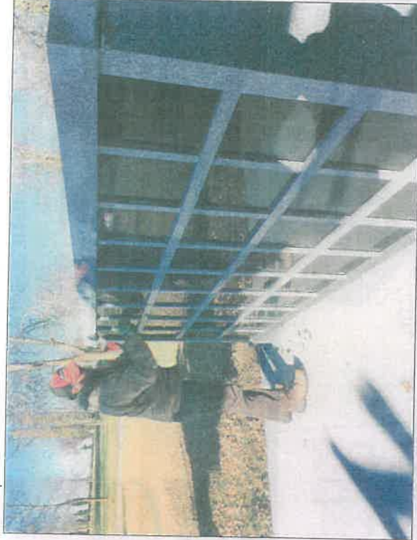
A crew from Fergus Falls Monument and Korby Contracting of Fergus Falls set a columbarium into place at the Wadena Cemetery Monday, Oct. 22. The new structure is weather proof and has 36 niches on each side, each able to hold up to two urns.
